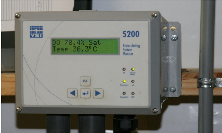
One of 20 wall-mounted 5200's on a grow-out tank.
